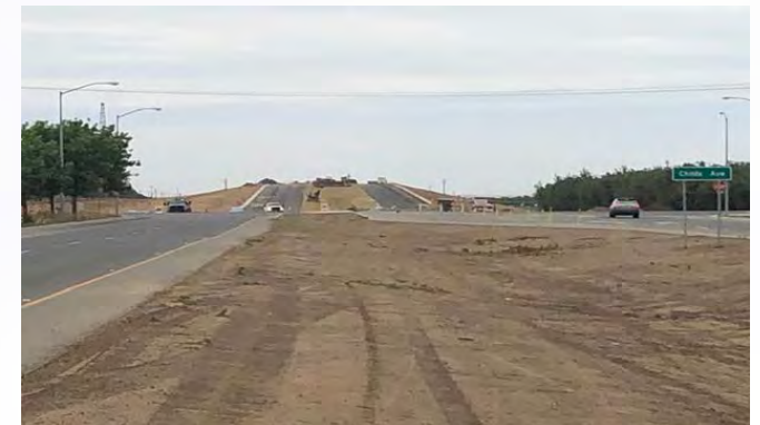
Campus Parkway Segment II, looking north from Childs Ave to Hwy 140 (May 15th, 2019)
